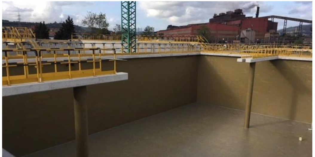
Chemical protection for reinforced concrete tanks using MasterSeal 7000 CR system (Asturias Spain)
