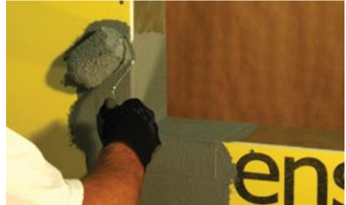
Step 4 Completely saturate the QUICK CORNER 6 with BASF fluid-applied air/water-resistive barrier material.
