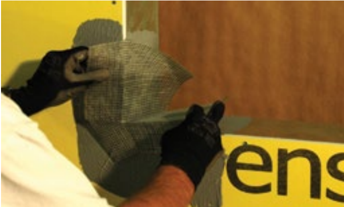
Step 3 Place the QUICK CORNER 6 on the BASF fluid-applied air/water-resistive barrier material.
