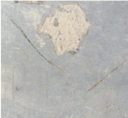
Figure 1 Top surface of a fragment removed from a warehouse slab that is delaminating
