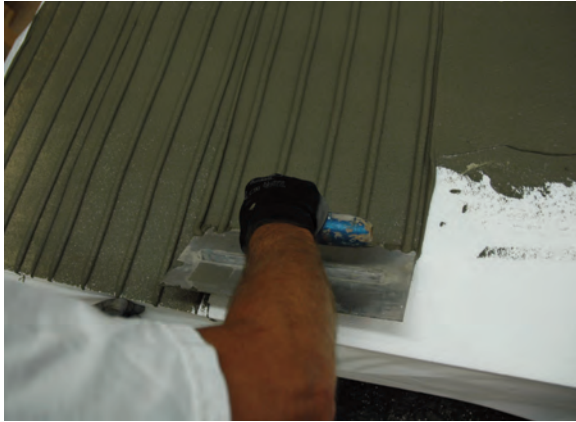
Cementitious adhesive/basecoat properly applied in vertical ribbons to back of EPS board.
