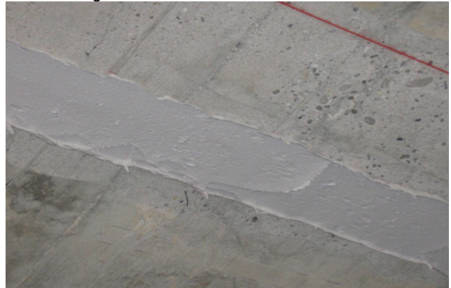
Figure 2. MasterBrace ADH 4000 is applied on to the concrete surface by using a steel spatula.
