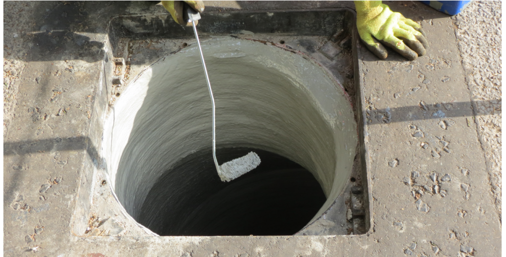
Our reference in Norwich (United Kingdom): Waste Water Manhole Chamber
