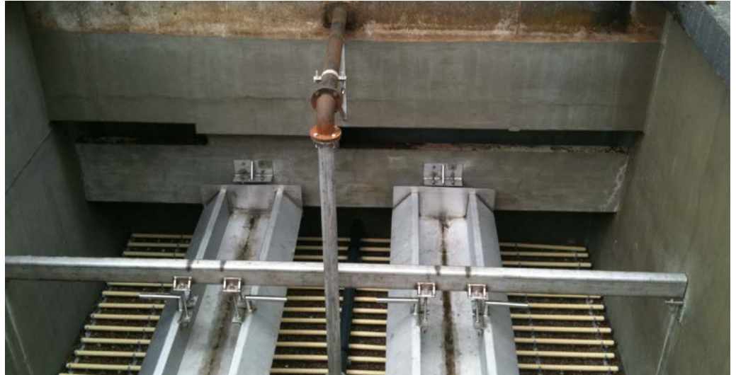
Our reference in West Wales (United Kingdom): Sluvad Water Treatment Works
