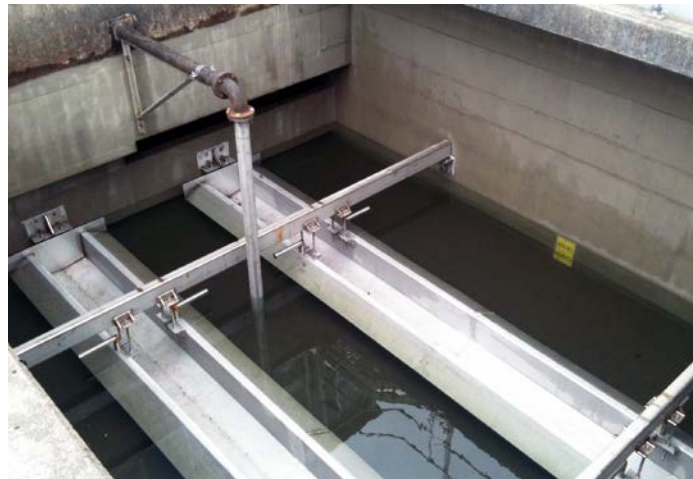
Our reference in West Wales (United Kingdom): Sluvad Water Treatment Works
