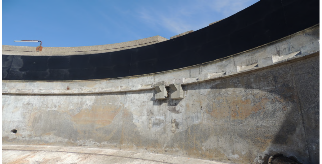
Our reference in London (United Kingdom): Sewage Treatment Works
