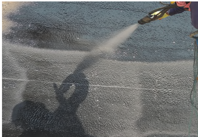
Our reference in London (United Kingdom): Sewage Treatment Works
