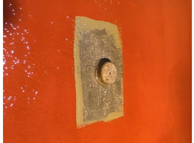
MasterSeal M 790 is applied in two coats - first in gray and then in red
