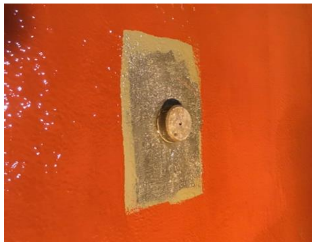
MasterSeal M 790 is applied in two coats - first in gray and then in red
