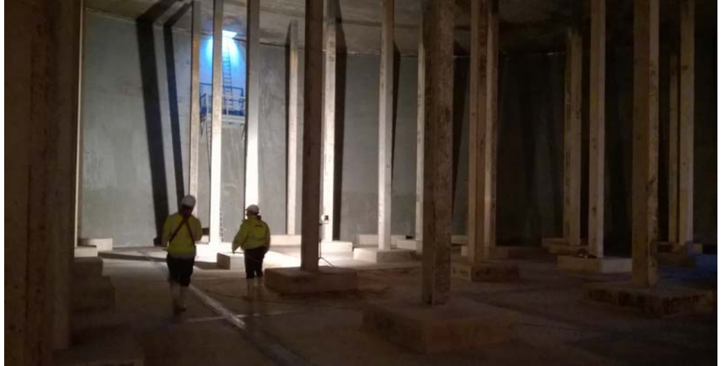
Our reference in Eastbourne (United Kingdom): Meades Service Reservoir No.1
