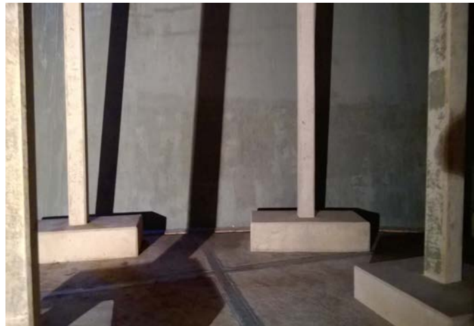
Our reference in Eastbourne (United Kingdom): Meades Service Reservoir No.1
