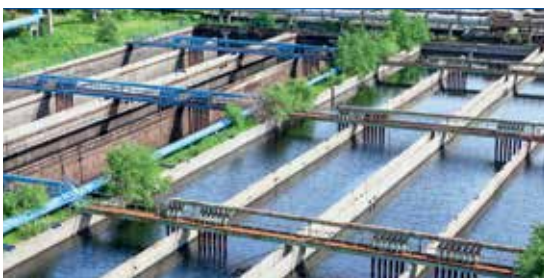
Tank for industrial process water
