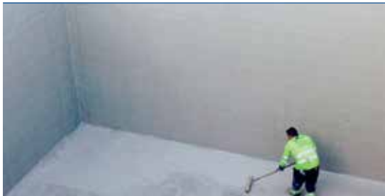
Process water reservoir, Montejo (Salamanca - Spain)
