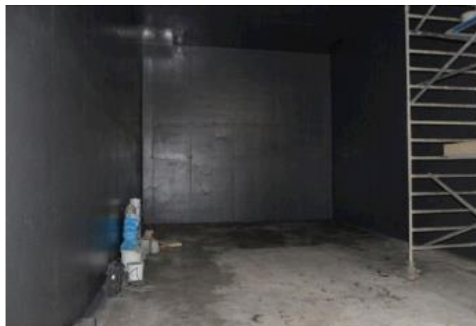
Our reference in Wavre (Belgium): Waterproofing and Protection of a Neutralization Basin
